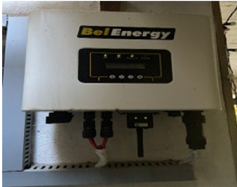
Figura 3 - Inversor Belenergy 4kW.
